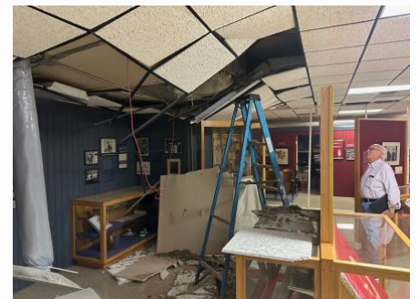
Damage to the ceiling tiles and rafters in the Coppock Wing of the museum
